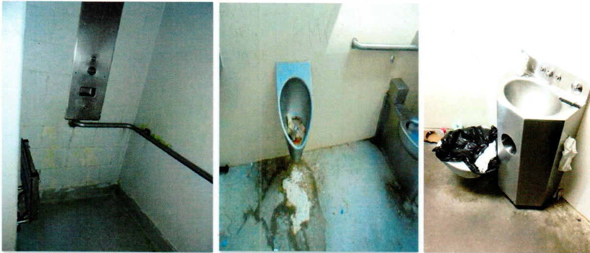
Figure 4. Shower stall with mold, mildew, and peeling paint (left). Outdoor recreation area with stuffed and overflowing toilet (center). Observed by OIG at the Adelanto facility on May 1, 2018. Detainee bathroom with mold and non-working toilet (right). Observed by OIG at the Essex facility on July 24, 2018. Source: OIG
